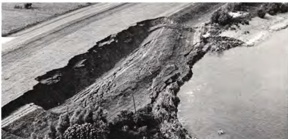
Levee slide showing a 700-foot section of the left (east) bank, Mississippi River levee which slid into the river on August 23, 1983 near Darrow, Louisiana after a recent high-water season.
