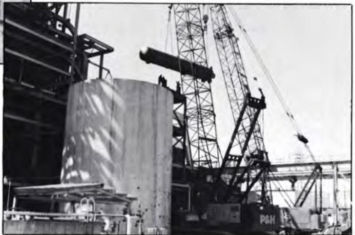
Heat exchanger for a power plant at Michoud, Louisiana.
